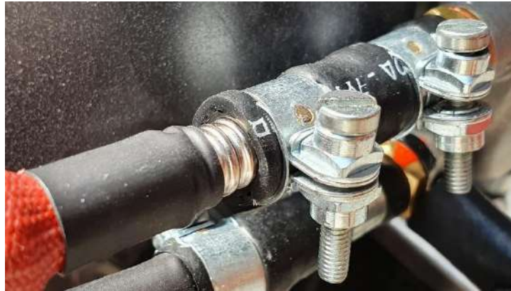
Figure 6: Fuel hose on corrugated pipe
