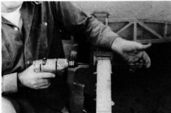
Photo No. 2: Bolt hole drilled straight through spar.
