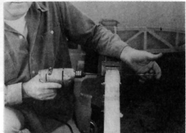
Photo No. 2: Bolt hole drilled straight through spar.
